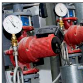
Sensors, valves and control cabinets
