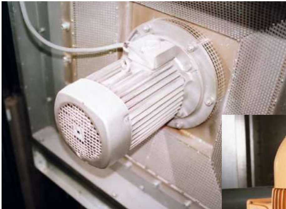
Monitoring a motor in a cooling system
