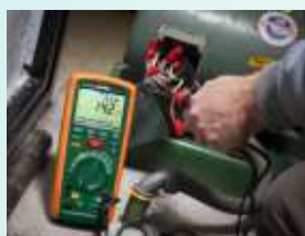
Insulation test on pump motor
