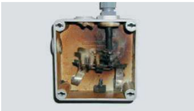
Module box after lightning strike
