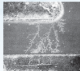
Corrosion you CAN'T see (what lies beneath)
