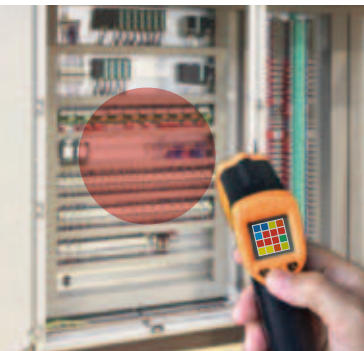
Transformers & distribution boards
